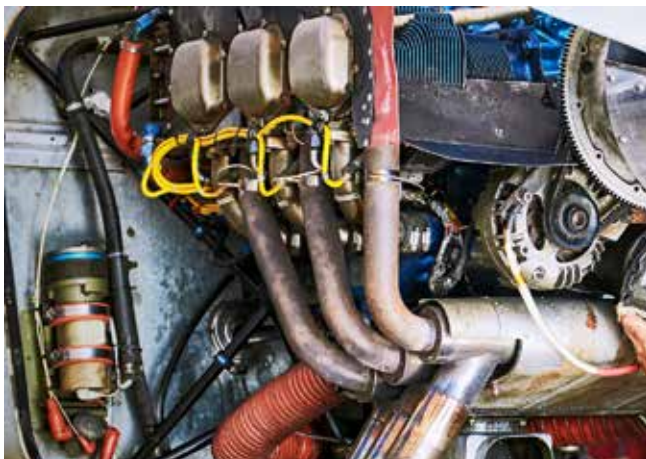
The muffler surrounding the exhaust pipes is the potential source of CO leaks (iStock/Bondariev)
